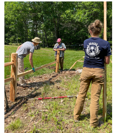
FLT staff and volunteers install a new split rail fence in the Morrill-Stillings Bird Sanctuary parking lot
